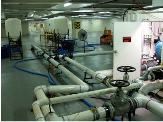
Test facilities of the Maritime Environmental Resource Center, onboard the M/V Cape Washington in the Port of Baltimore.
